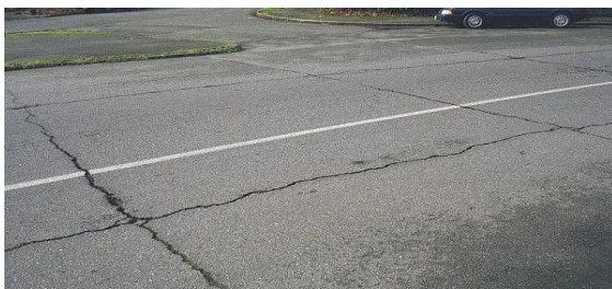
Gambar 10. Longitudinal & Transversal Cracking
