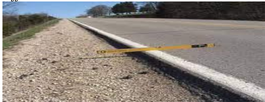
Gambar 9. Lane/Shoulder Drop Off
