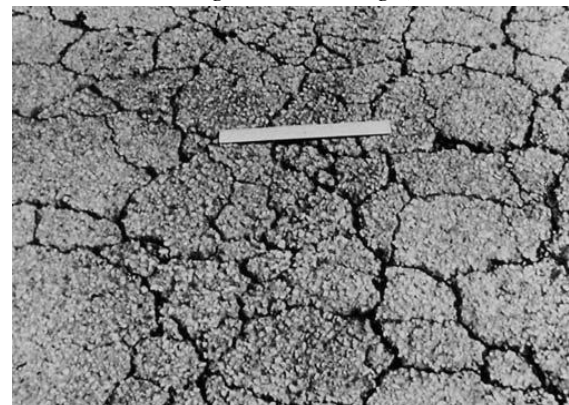
Gambar 1. Alligator Cracking (Retak Kulit
